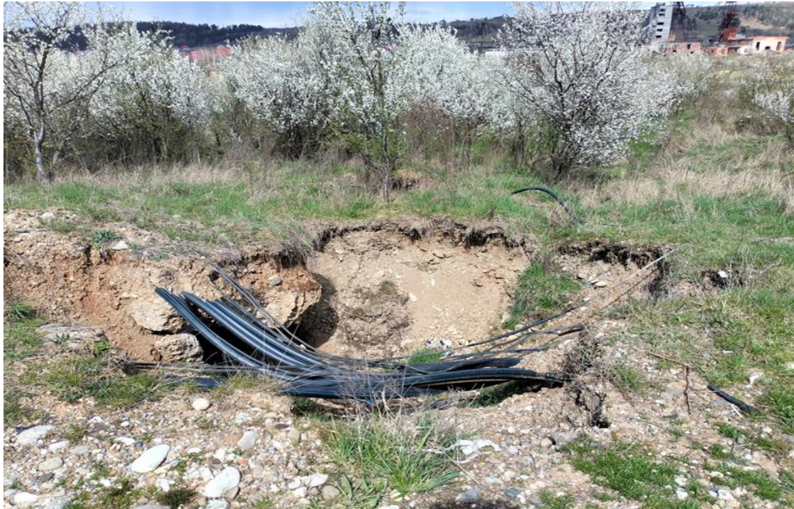
Figure 3 F. New sinkholes to the west of mine funnel #7 (Photo 2023-04-10)
