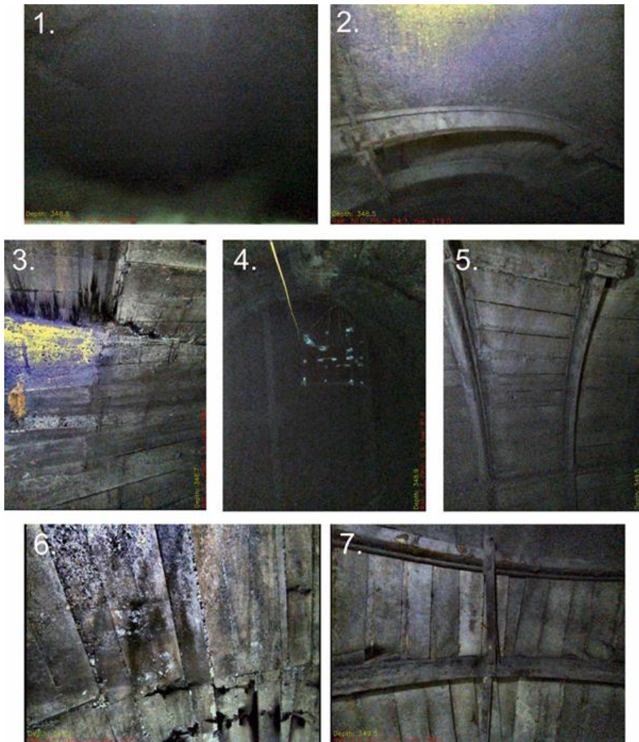
Figure 47 - Visual image of the side passage at 366 m. 1. front camera view of the entrance; 2. front camera view of the concrete entrance; 3. side camera view of the concrete side of the entrance; 4. side camera view of the shaft and the safety cage; 5. side cam
