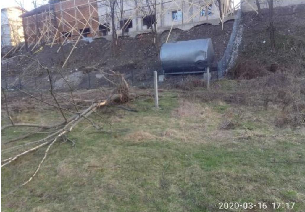
Figure 3 A. The body of the flood-control dam continues to be actively built up, with the clearing of woody vegetation, the arrangement of open drainage of sewage water into a drainage trench (Photo 2020-03-16)
